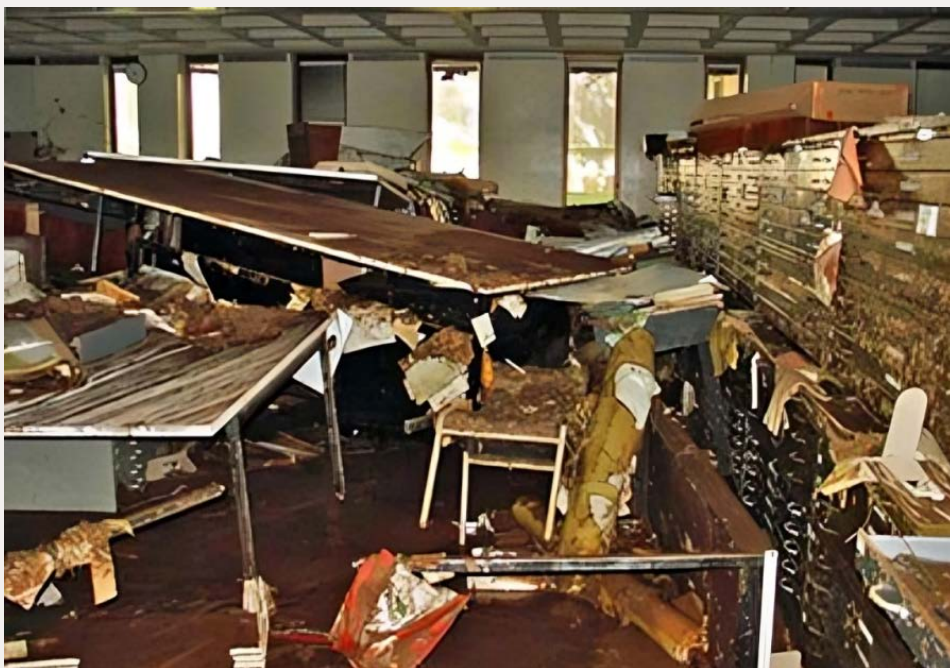
The flood-damaged map collection on the ground floor of Hamilton Library in 2004 28
